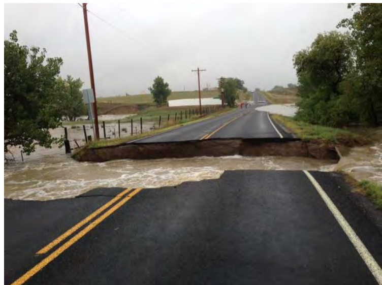
FIGURE 30. DAMAGES FROM 2013 FLOOD EVENT
