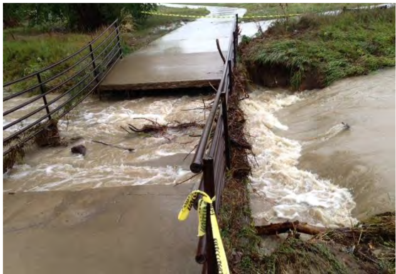
FIGURE 1. DAMAGES FROM 2013 FLOOD EVENT
