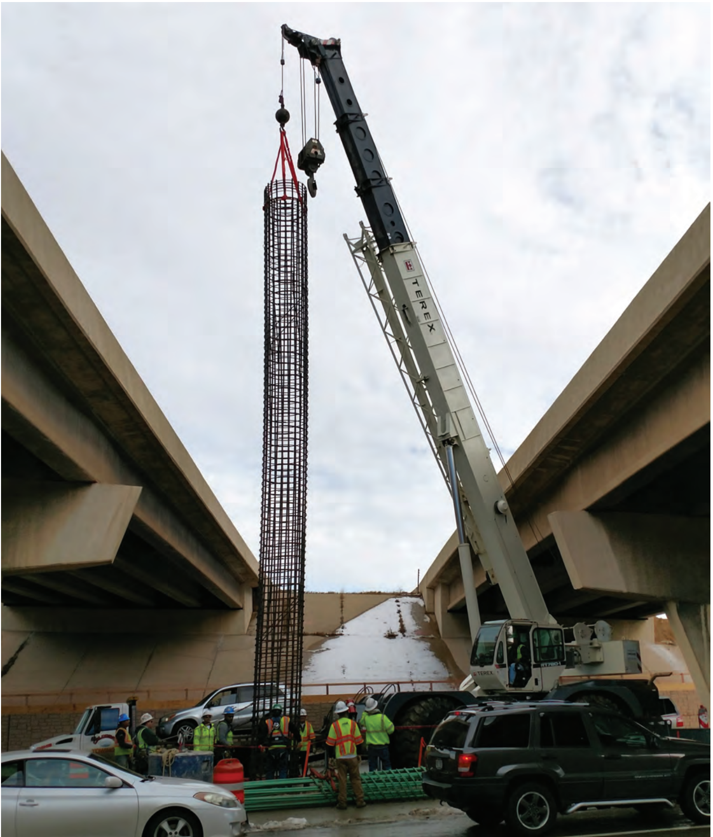
The Colorado Department of Transportation conducts foundation work at Broadway for bridge widening as part of the C-470 Express Lanes project. More than 100,000 motorists daily use the section of C-470 between Interstate 25 and Wadsworth Boulevard.
