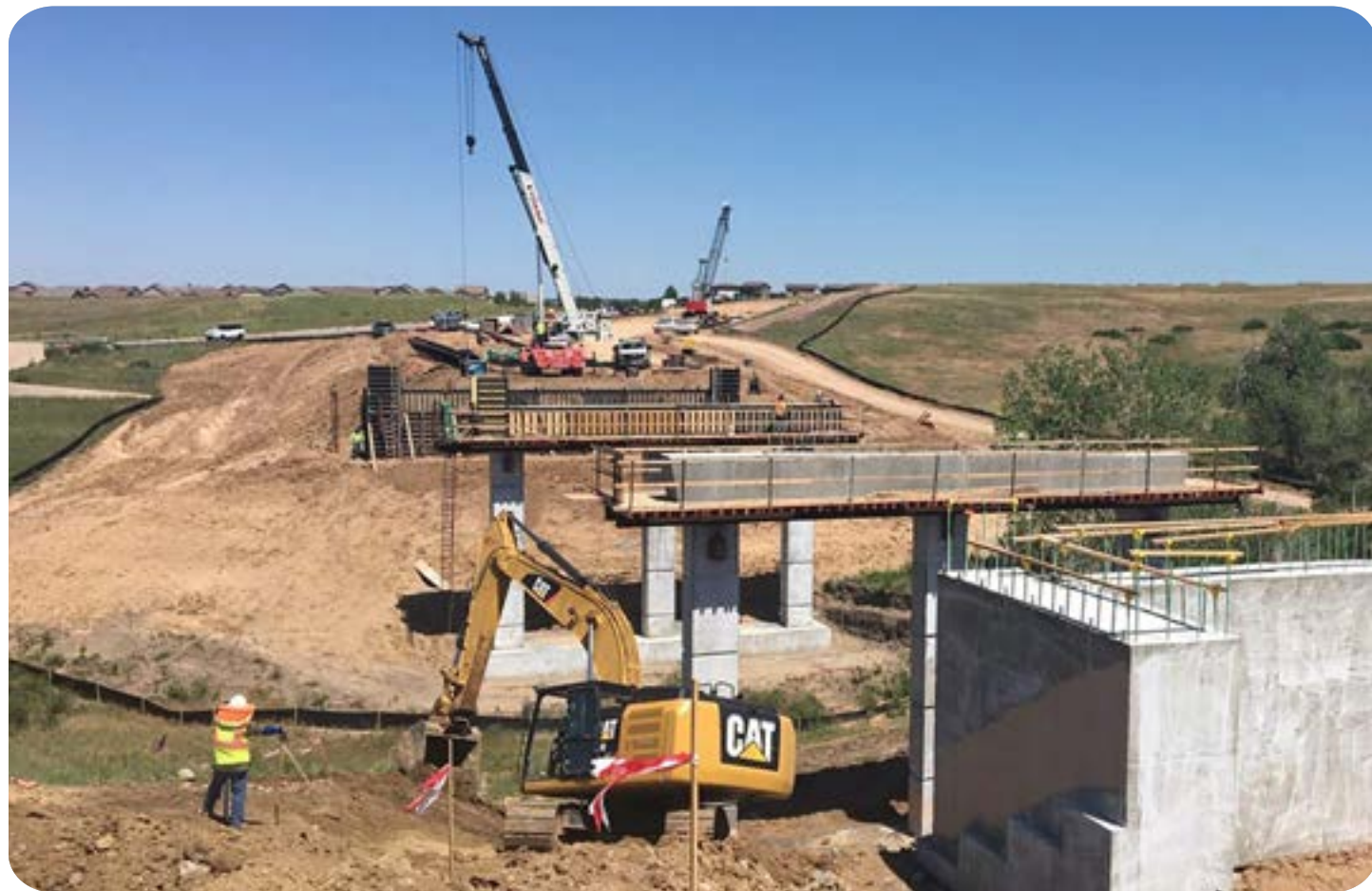
Of the 3,116 bridges in the Denver region, 45 are considered to be in poor condition. Maintenance and reconstruction activities improve the quality of bridges throughout the region, including along RidgeGate Parkway in Lone Tree. Photo courtesy of the City of Lone Tree.
