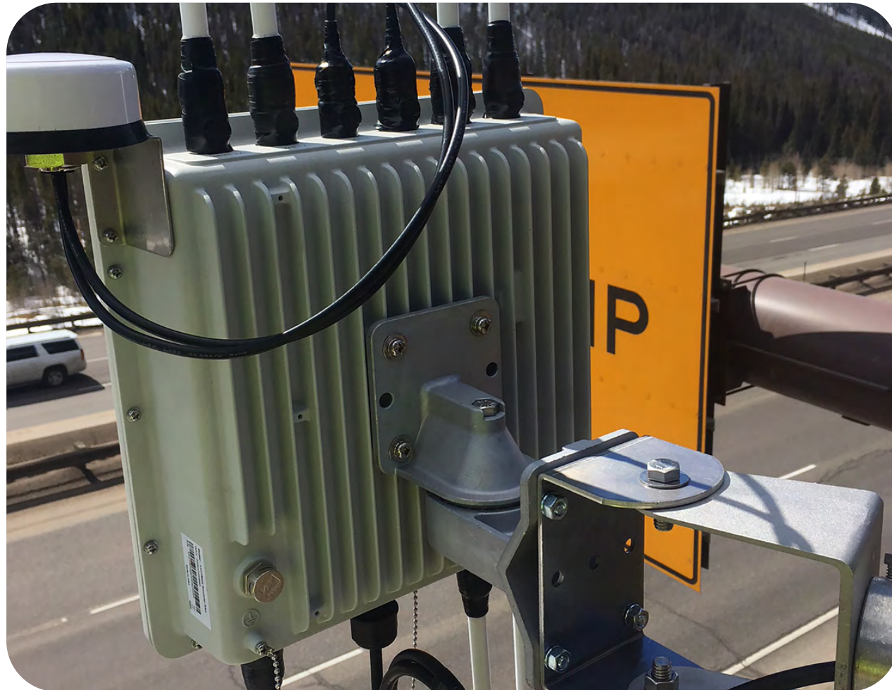
Infrastructure can communicate with and send alerts to connected vehicles. Photo credit: CDOT
