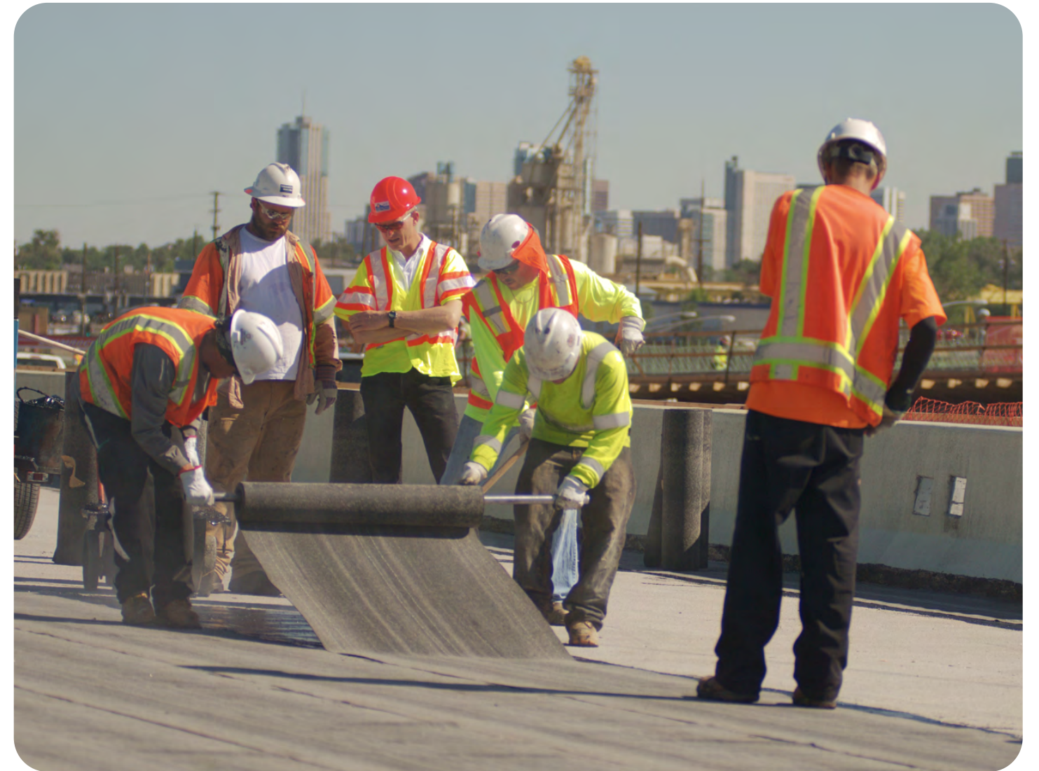
Nearly half of CDOT's annual budget goes to maintaining the existing system. Photo credit: CDOT
