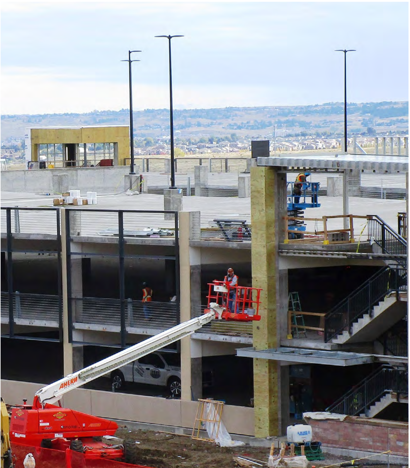
When completed, RidgeGate Parkway station at the southern end of the Regional Transportation District's Southeast Rail Extension will include a 1,300-space park-and-ride facility. The station is just one example of the continuing expansion of the region's rapid transit system.
